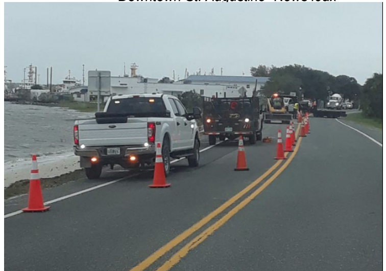
Tidal Surge undermining A1A in Mayport- FDOT on scene
